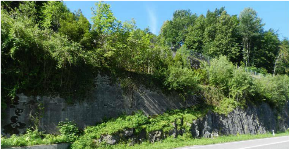
Figure 6. Double gravity wall (note the fence demarcating the crest of the upper wall)
